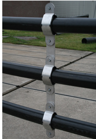
TYPICAL INSTALLATION, PHOTO TAKEN AT A SHORT CIRCUIT TESTING EVENT AT KEMA LAB, ARNHEM NL.
