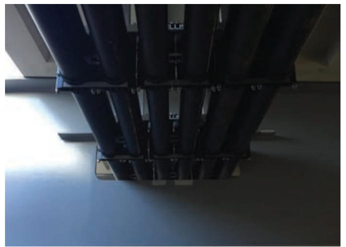
Duct support under a road bridge
