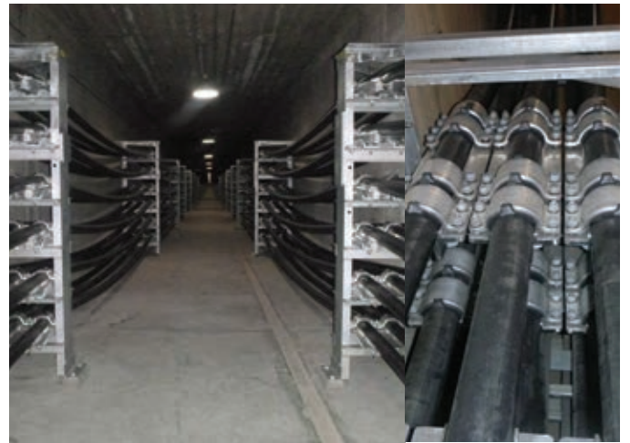
Fort Randall, cable saddles in hydro electric dam
