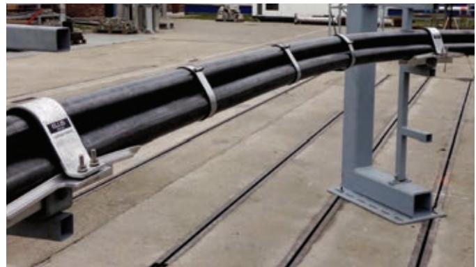
A photo of the short circuit test rig for centaur trefoil including flexi-straps. Testing was carried out at ZKU Laboratories in Prague, CZ.
