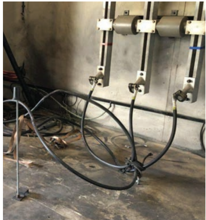
Short circuit testing What happens when cables are not cleated (only straps were used)
