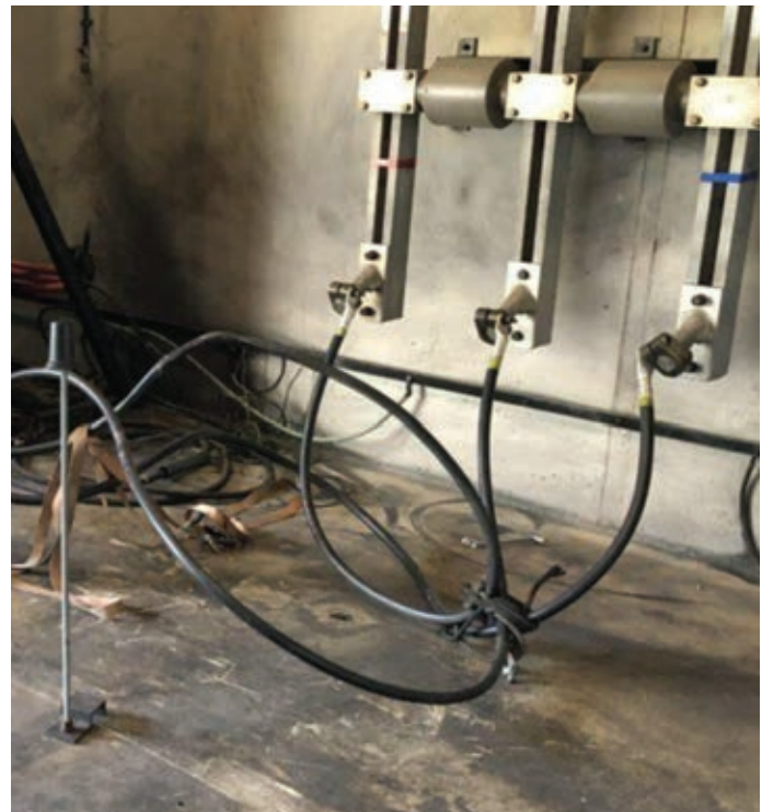
Short circuit testing What happens when cables are not cleated (only straps were used)
