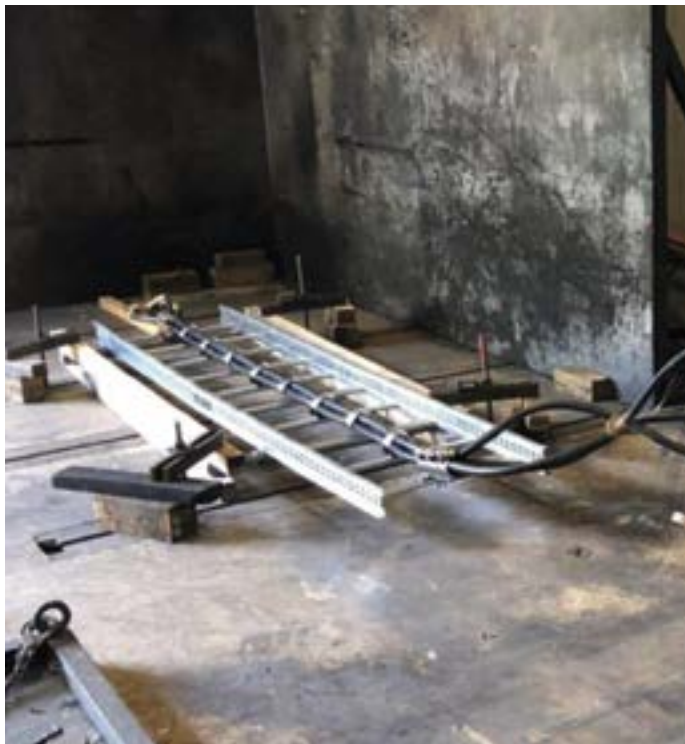
Short circuit testing Correctly cleated cables
