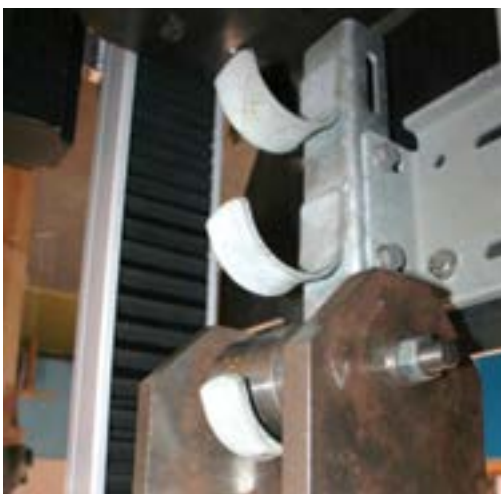
Cable hangers for London Underground
