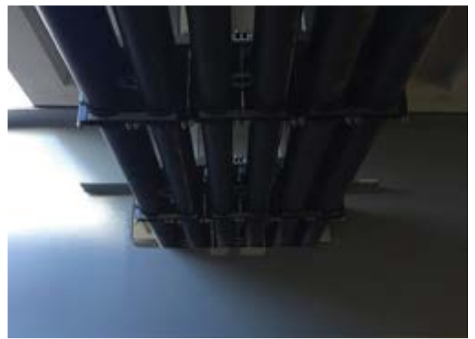
Duct support under a road bridge
